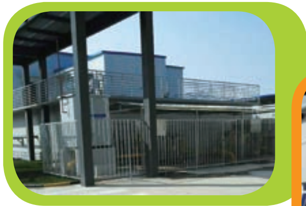
鍋爐燃氣調控站 Boiler gas control station
